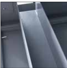
Enclosed cable ducting
