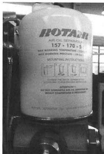
Figure 13.4-7 Oil separator filter
